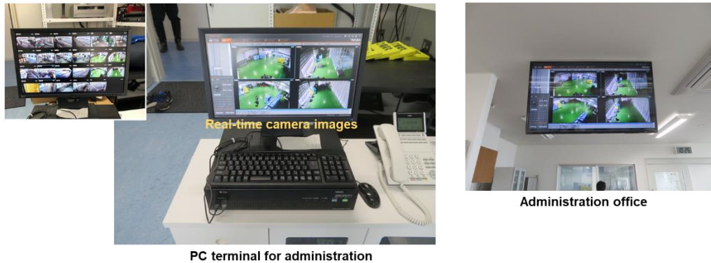
Figure 4.3 Surveillance cameras installed throughout the fishing port, Akkeshi, Japan
